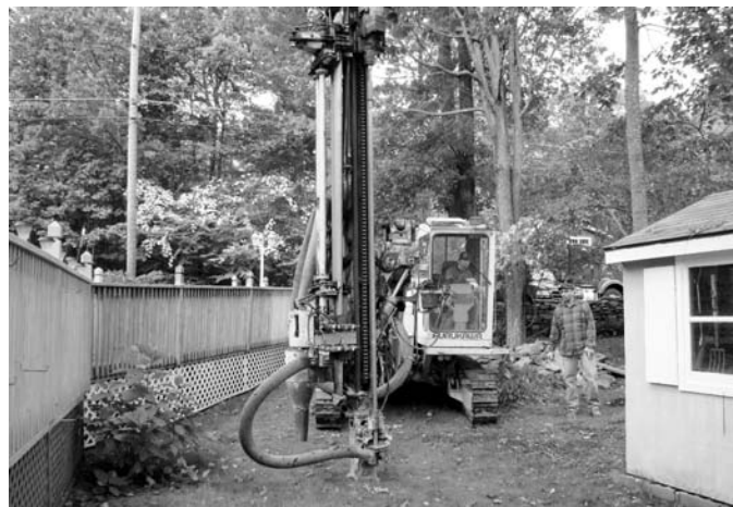
ABOVE: Drilling rig sets up for first of five wells. BELOW: Side yard after drill rig and excavator were finished and surface rough-graded.
